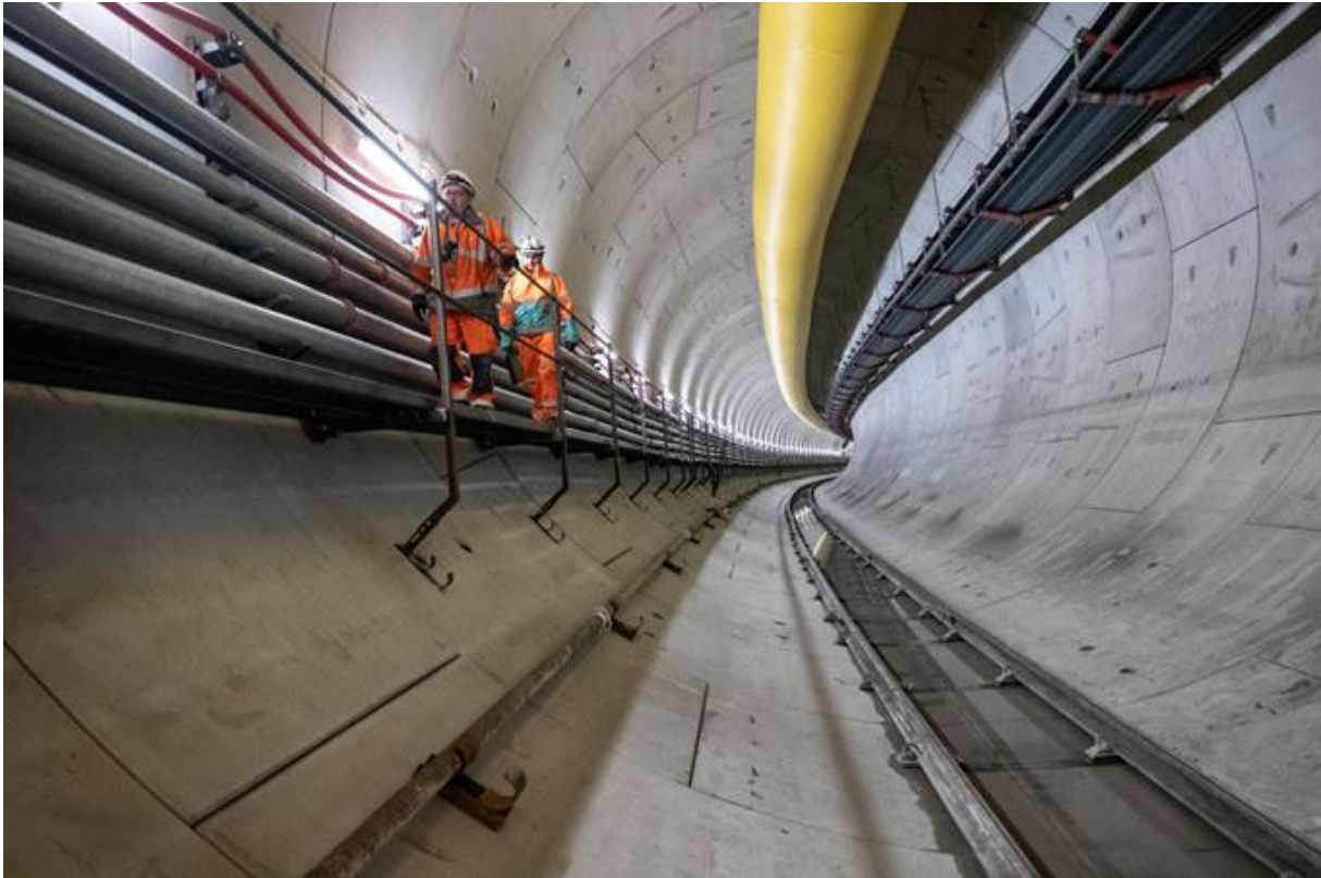
Figure C8: Concrete segmental lined tunnel during construction (© Crossrail Ltd) Note: walkway, cables & pipework (left), ventilation duct (top) and conveyor (upper right)
