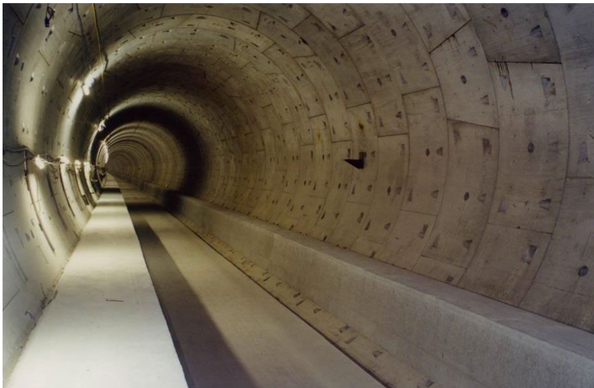
Figure C9: Finished 7.15m internal diameter segmentally lined permanent tunnel (© Channel Tunnel Rail Link)
